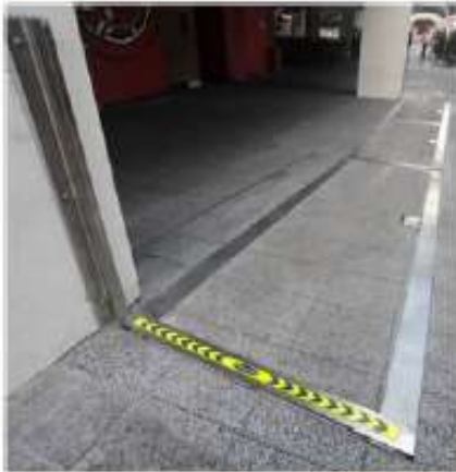
Tanglin Mall flood gates - flat
