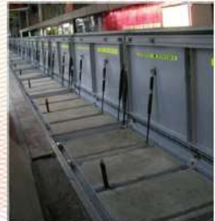
Lucky Plaza flood gates - activated
