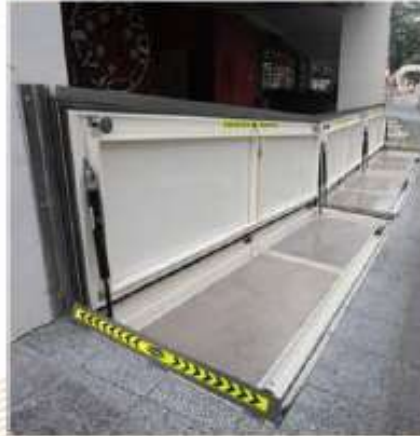
Tanglin Mall flood gates - activated
