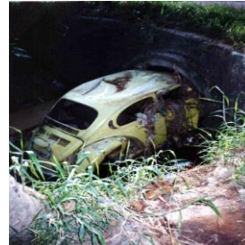
Flow obstruction from solids 4
