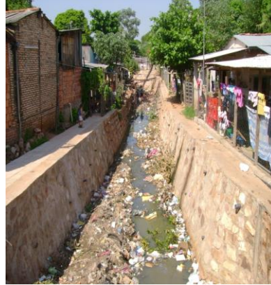
Integrated impacts: lack of water supply, sewage, drainage, solids and illegal occupation
