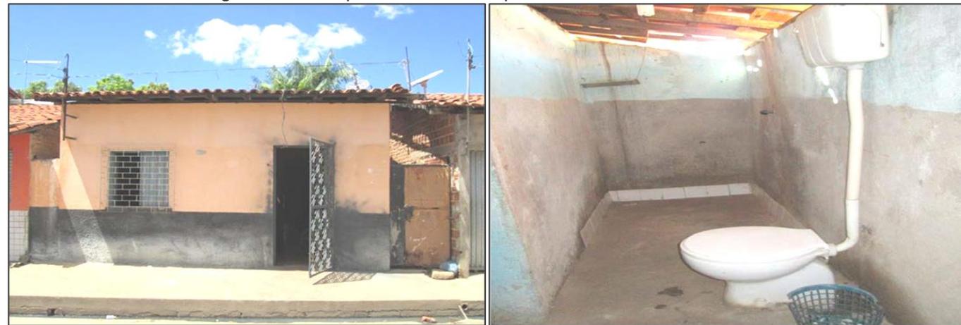
Figure 4. Example of a standard property estimated at 'Low' level. Left: façade. Right: bathroom without tile.
