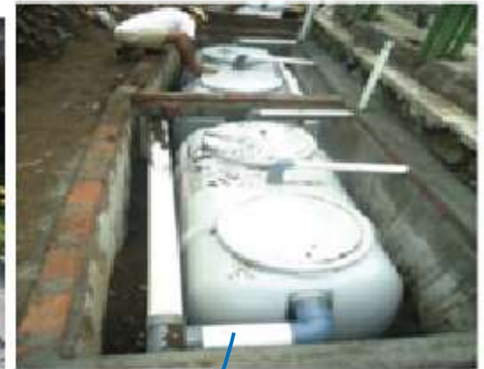
Biofill (communal septic tank)
