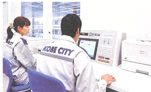
Radio Control Room
