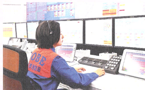
Fire Services Control Room
