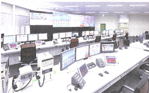
Fire Services Control Room general view
