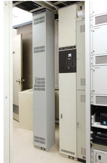
■ Disaster prevention administration radio system in the master station
