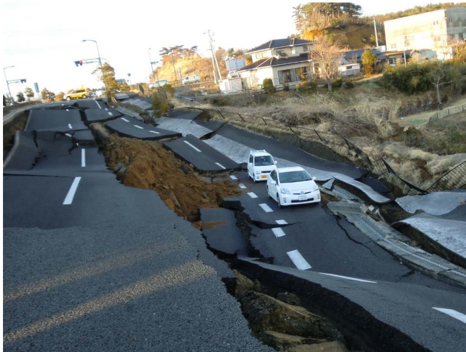
▲Route 6 was heavily damaged. Hirono Town, Fukushima Pref.
