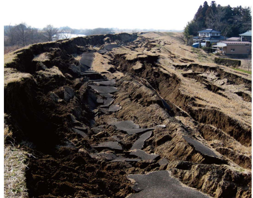
▲ Massive land sinking under Seawalls Left bank of Naruse river, Shimonakanome, Osaki City, Miyagi Pref.
