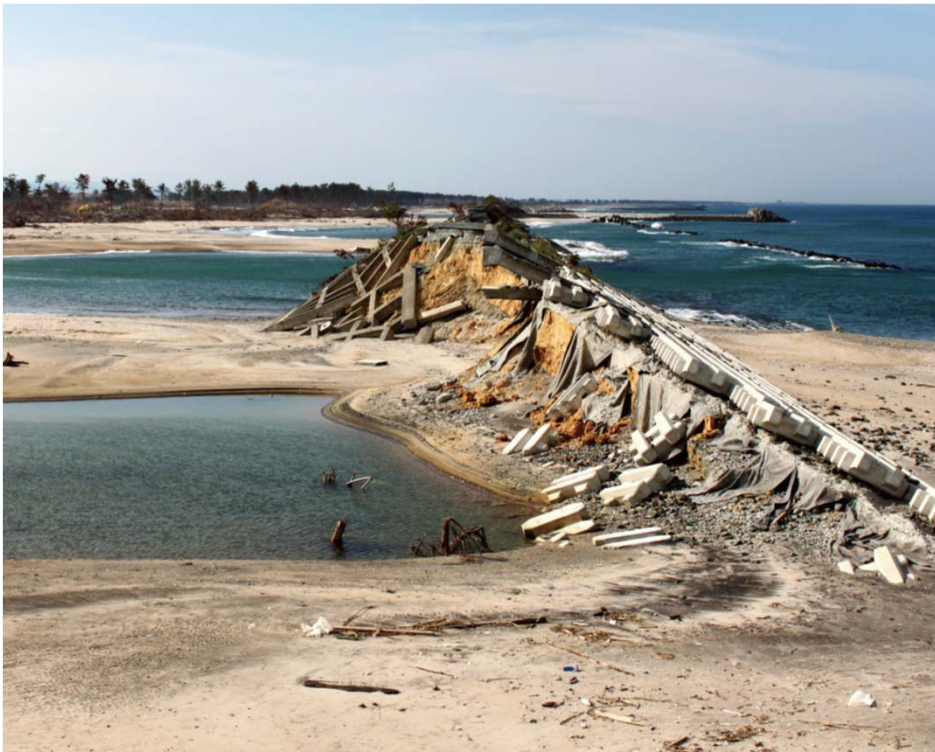
▲ Seawalls broken by tsunami Southern coastline of Sendai Bay Yamamoto Town, Watari Country, Miyagi Pref.
