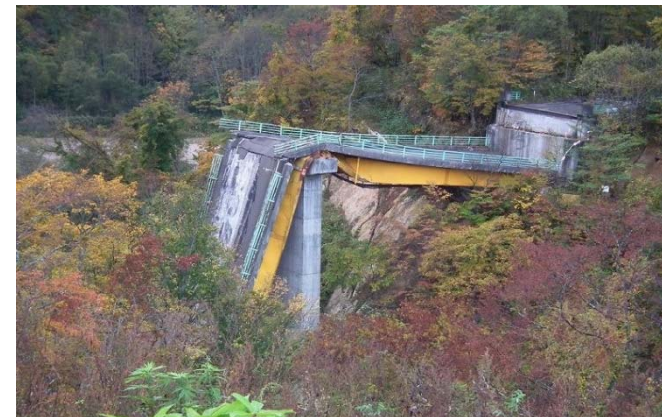
▲ Matsurube Bridge (Ichinoseki City, Iwate Pref.) (collapsed in the Iwate Miyagi Inland Earthquake in June, 2008)
