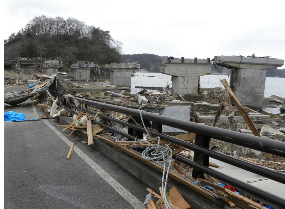
▲Bridge girders on Route 45 were completely swept away. Minamisanriku Town, Miyagi Pref.
