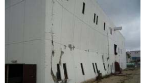
Damage of pumping facility
