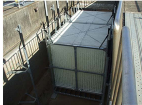
Temporary wastewater treatment by the contact oxidation process
