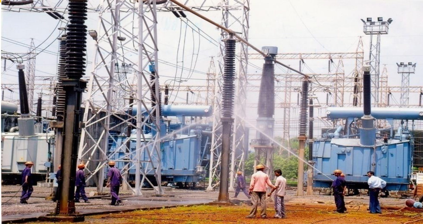
Demonstration of 400 kV live line insulator washing of Kalwa Sub – Station of Maha Transco Ltd., Mumbai.
