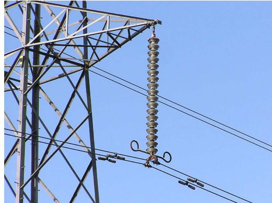
Insulators – ceramic or polymer separate conducting parts
