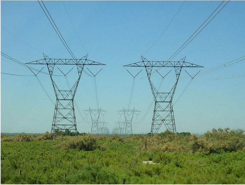
500 KV/3500MW AC transmission line (Southern California Edison)
