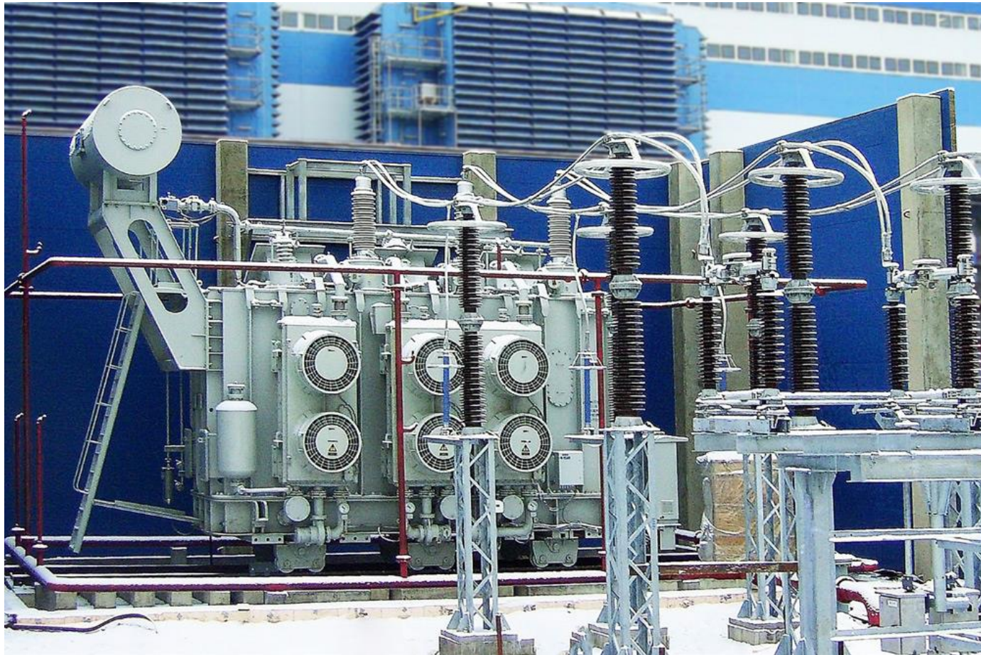
Generator Step-up Transformer Next To A Power Station (250MVA 15KV/110KV)
