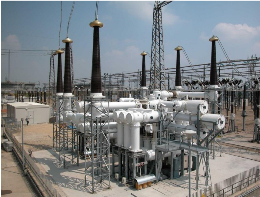
420 kV gas insulated switchgear
