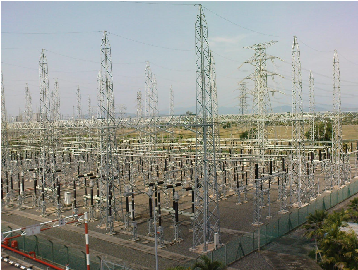
Switch Yard Next To A Power Plant (10.5KV/275KV, 168MVA station)
